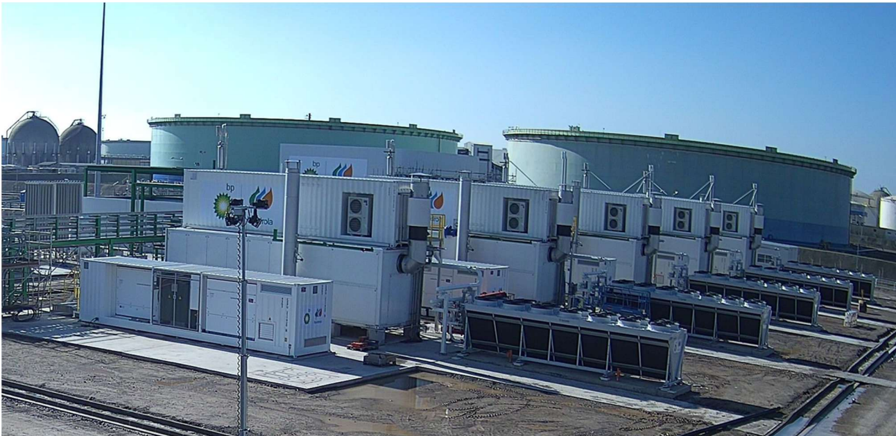
Progress on the hydrogen project at the bp refinery in Castellón, Spain
