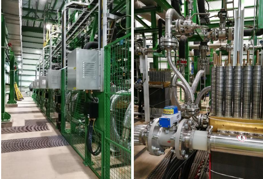
PEM technology 16 stacks of 1.25 MW each
