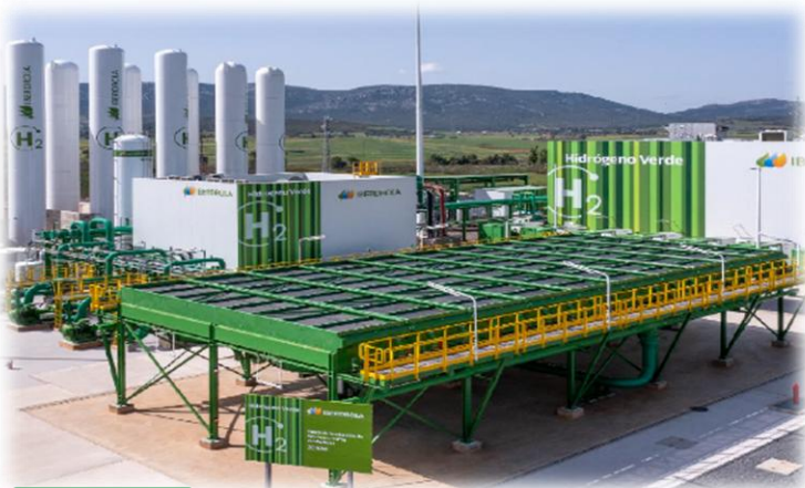
20 MW Green H 2 plant in Puertollano
