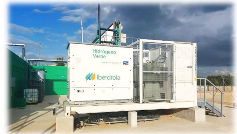
1.25 MW Green H 2 plant in Benicarló
