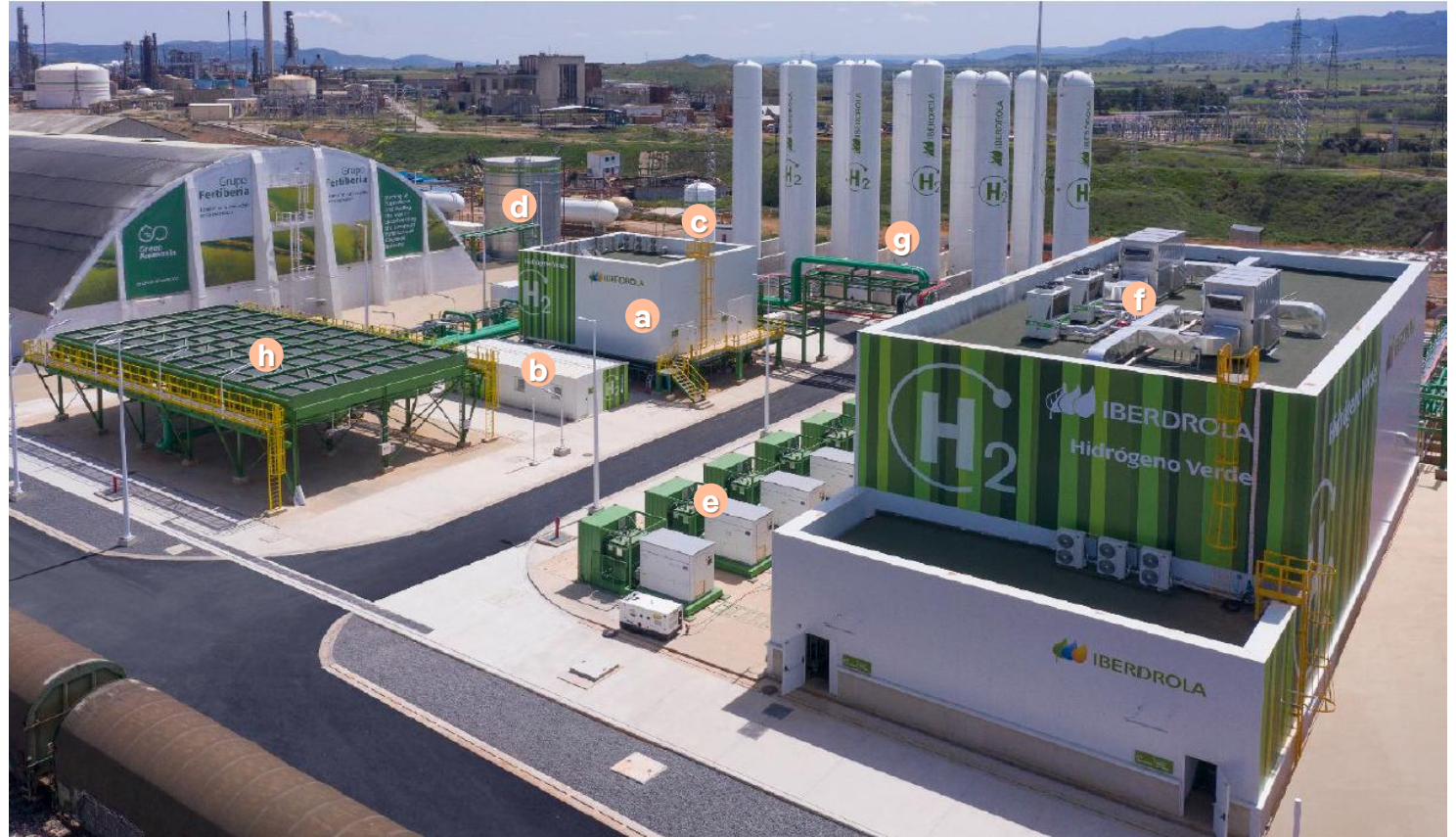
Compression system behind the electrolyzer building
